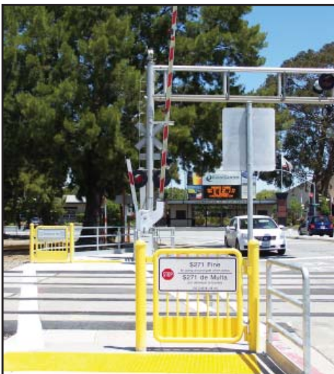
Grade crossing work at 25 th Avenue in San Mateo will be completed in late summer.
