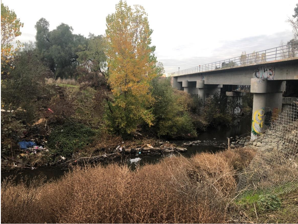
Photo 1. Looking downstream at Guadalupe MT-2 track bridge. Guadalupe River and associated riparian habitat are clearly visible.
