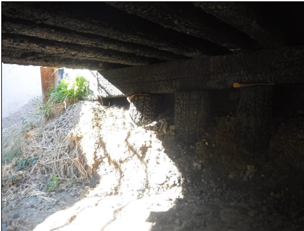
Photo 1: Abutment 1 – Typical fire damage and leaking ballast.
