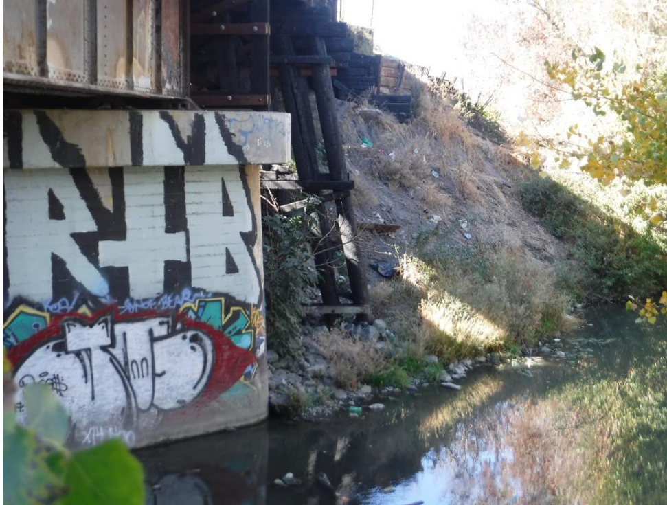
Photo 4: Failing channel protection on northeast embankment.
