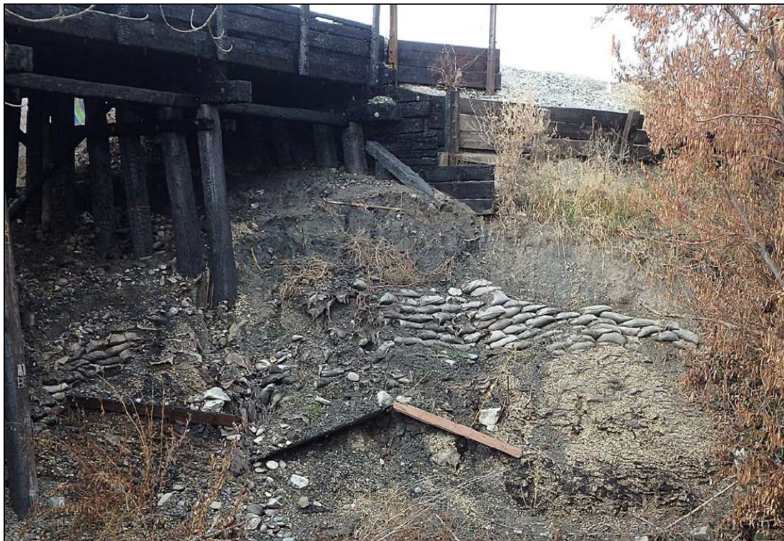
Photo 7: 2018 Condition of MT-1 bridge and left bank. Note fire damage to timbers and deterioration of temporary stabilization measures.
