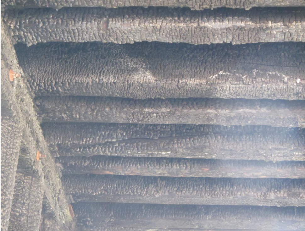
Photo 2: Typical stringer span fire damage.
