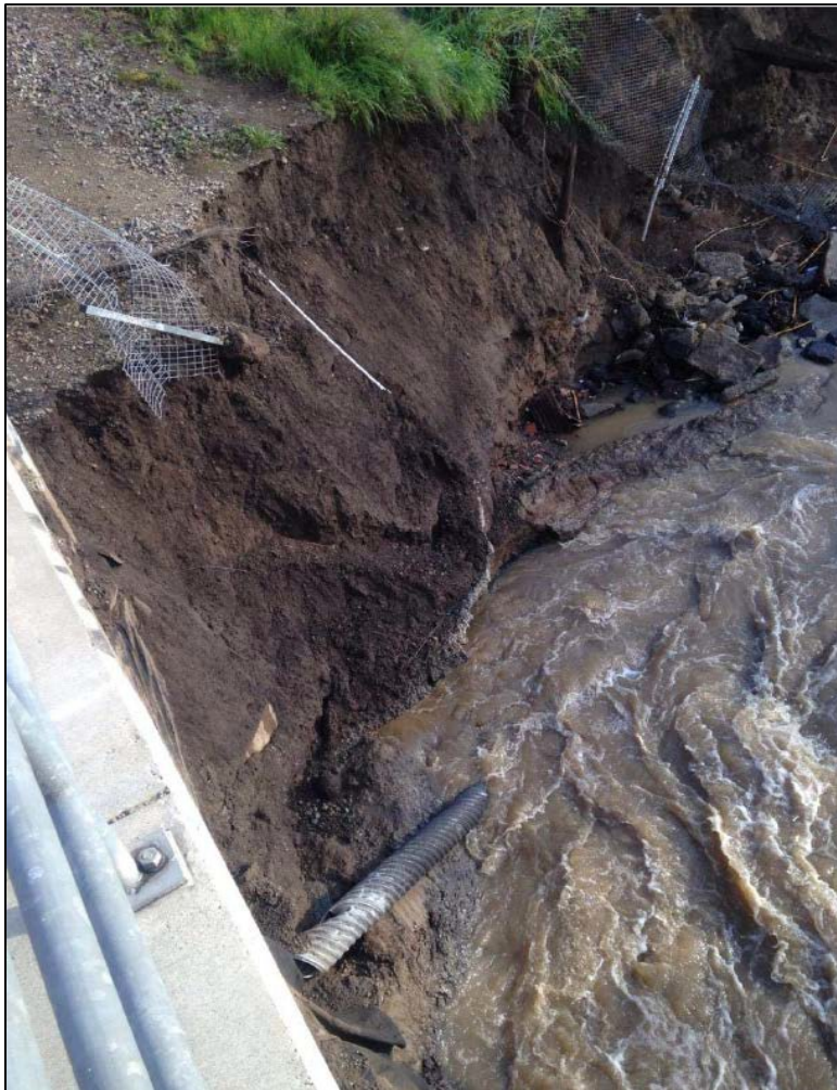
Photo 8: 2017 Bank failure at MT-2 that required emergency repairs.
