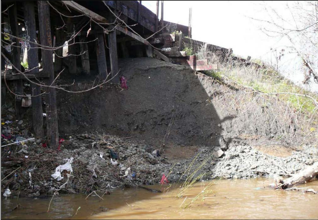
Photo 6: 2014 Bank failure at MT-1 downstream left bank required emergency repair.
