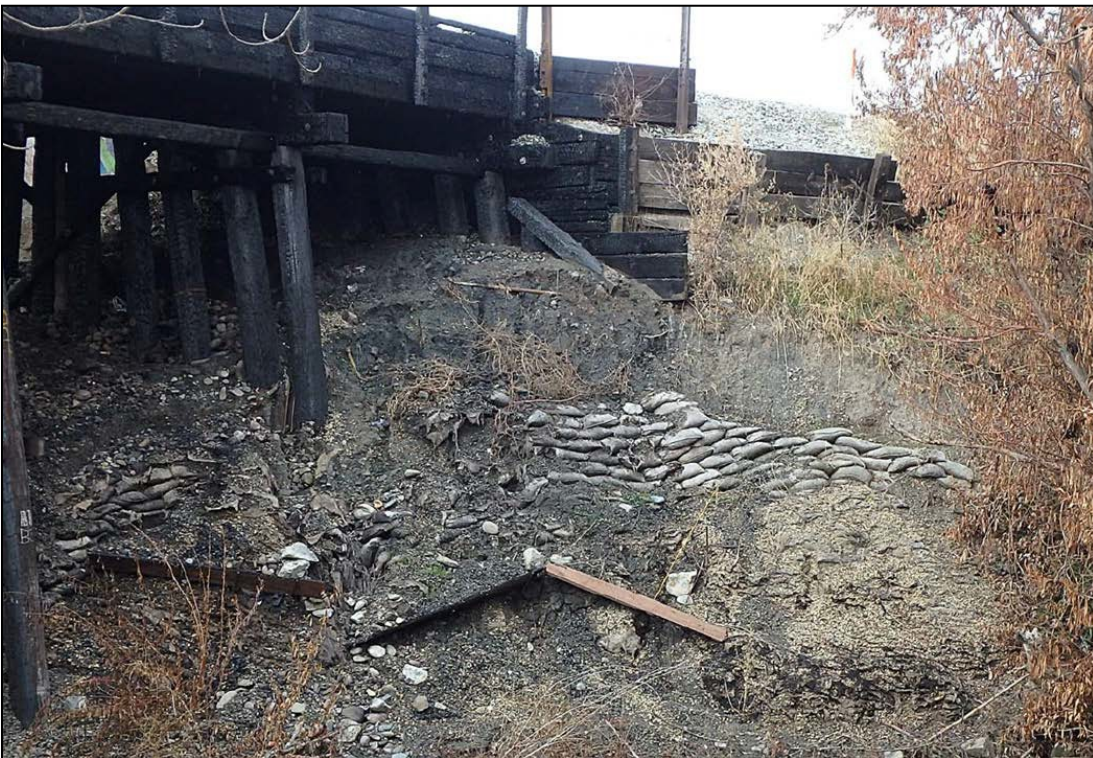
Photo 7: 2018 Condition of MT-1 bridge and left bank. Note fire damage to timbers and deterioration of temporary stabilization measures.
