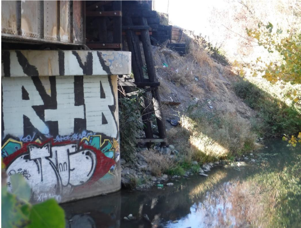
Photo 4: Failing channel protection on northeast embankment.
