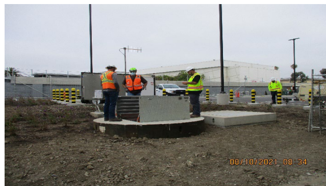
Photo 2 - Pump Station Testing
