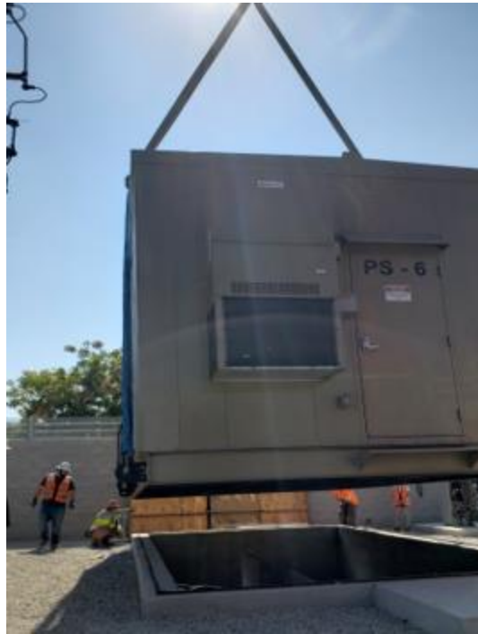
Set Control Building and Switchgear at PS-5, PS-6, and PS-7
