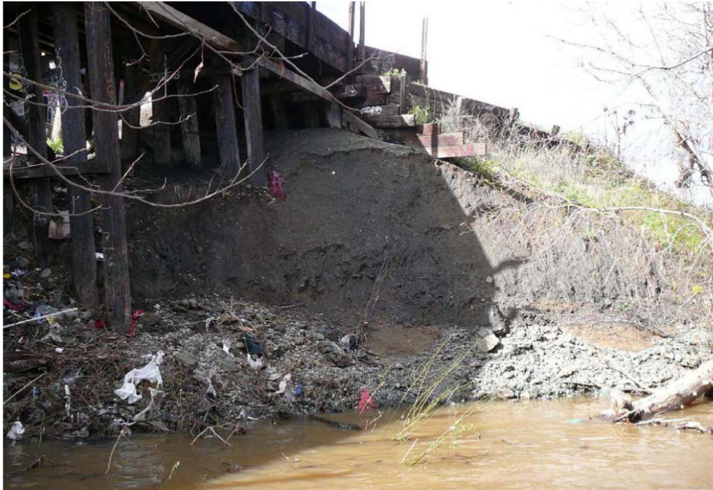
MT-1 Bank Failure
