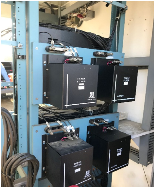
Photo 1 - New advance signal preemption equipment
