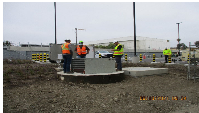
Photo 2 - Pump Station Testing
