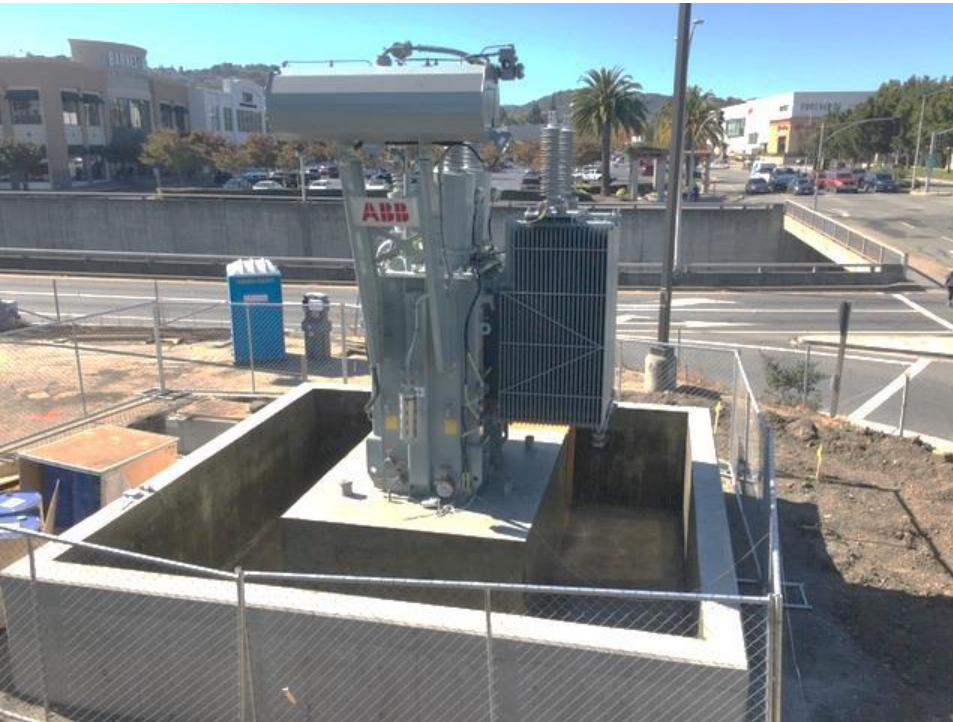
Paralleling Station 4 Hillsdale Station
