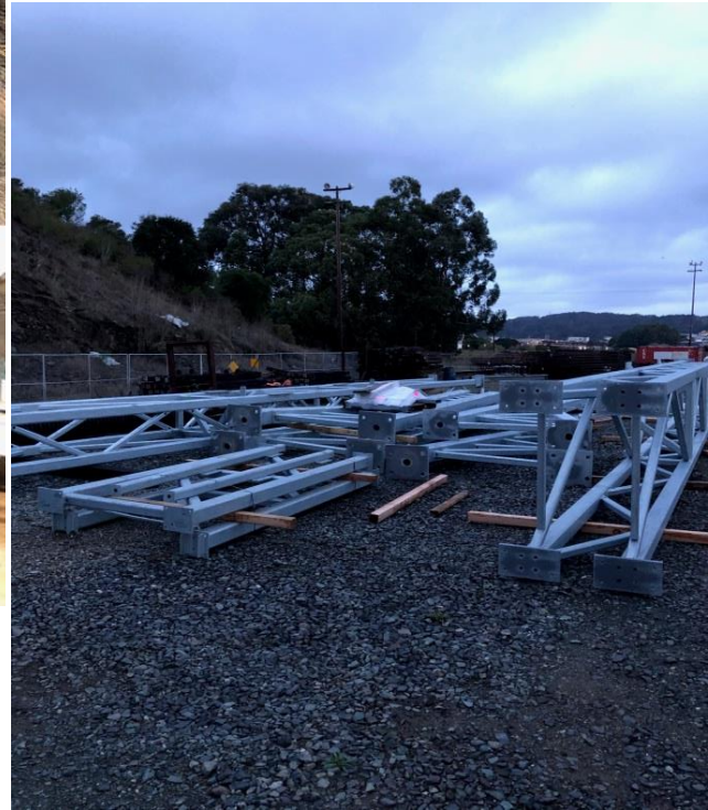
Tunnel 4 South OCS Termination Structure
