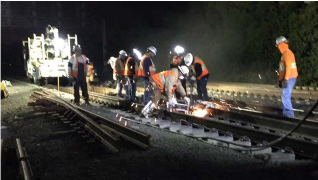
Track crew cutting the existing switch frog prior to removal. New switch frog is shown to the left.
