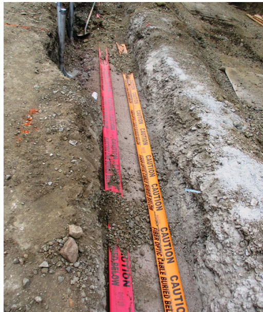
Identification tape placed above utilities
