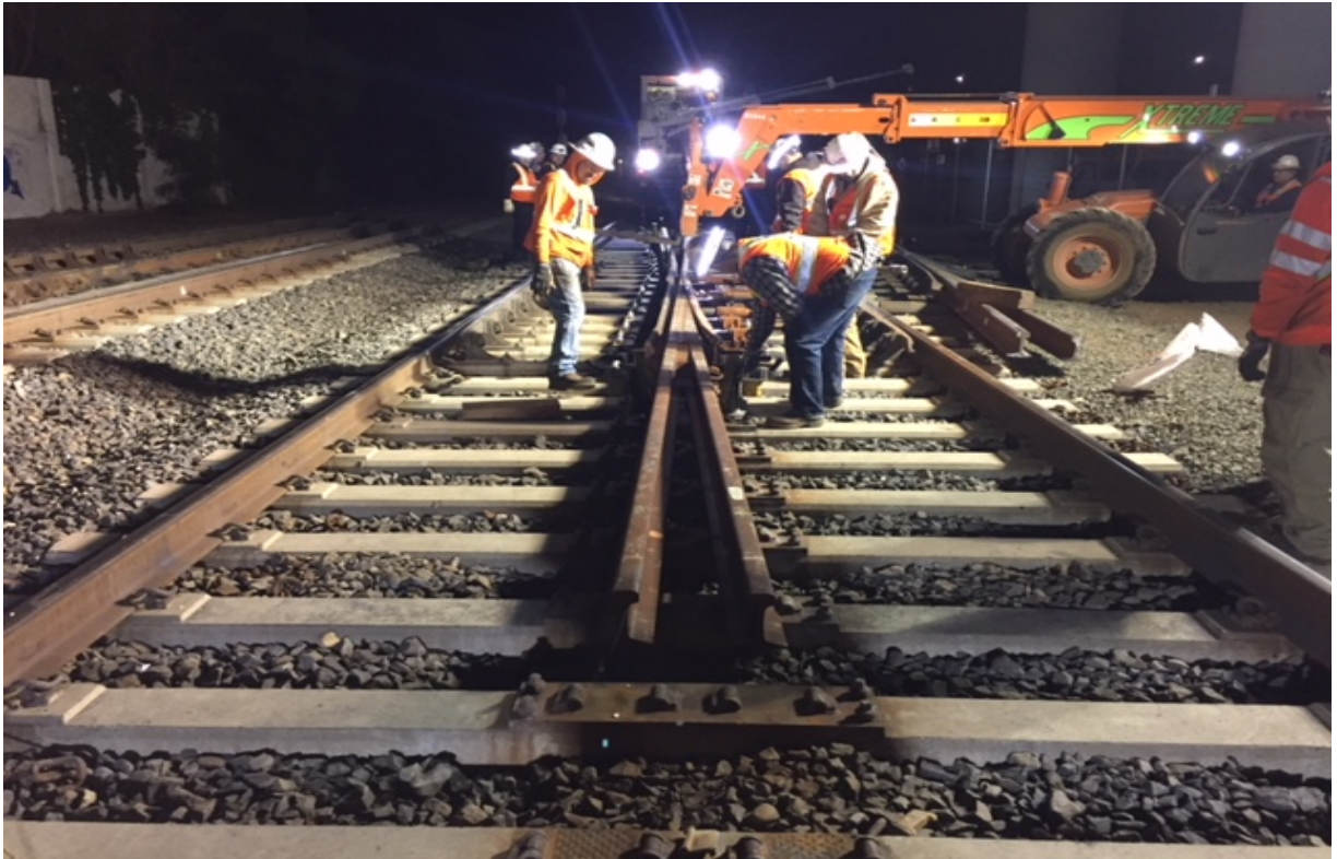
Track crew sets the new switch frog into place prior to installation of additional rail and clips.
