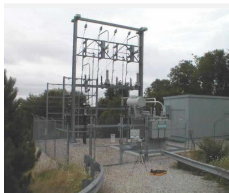
Paralleling Station - Amtrak Northeast Corridor
