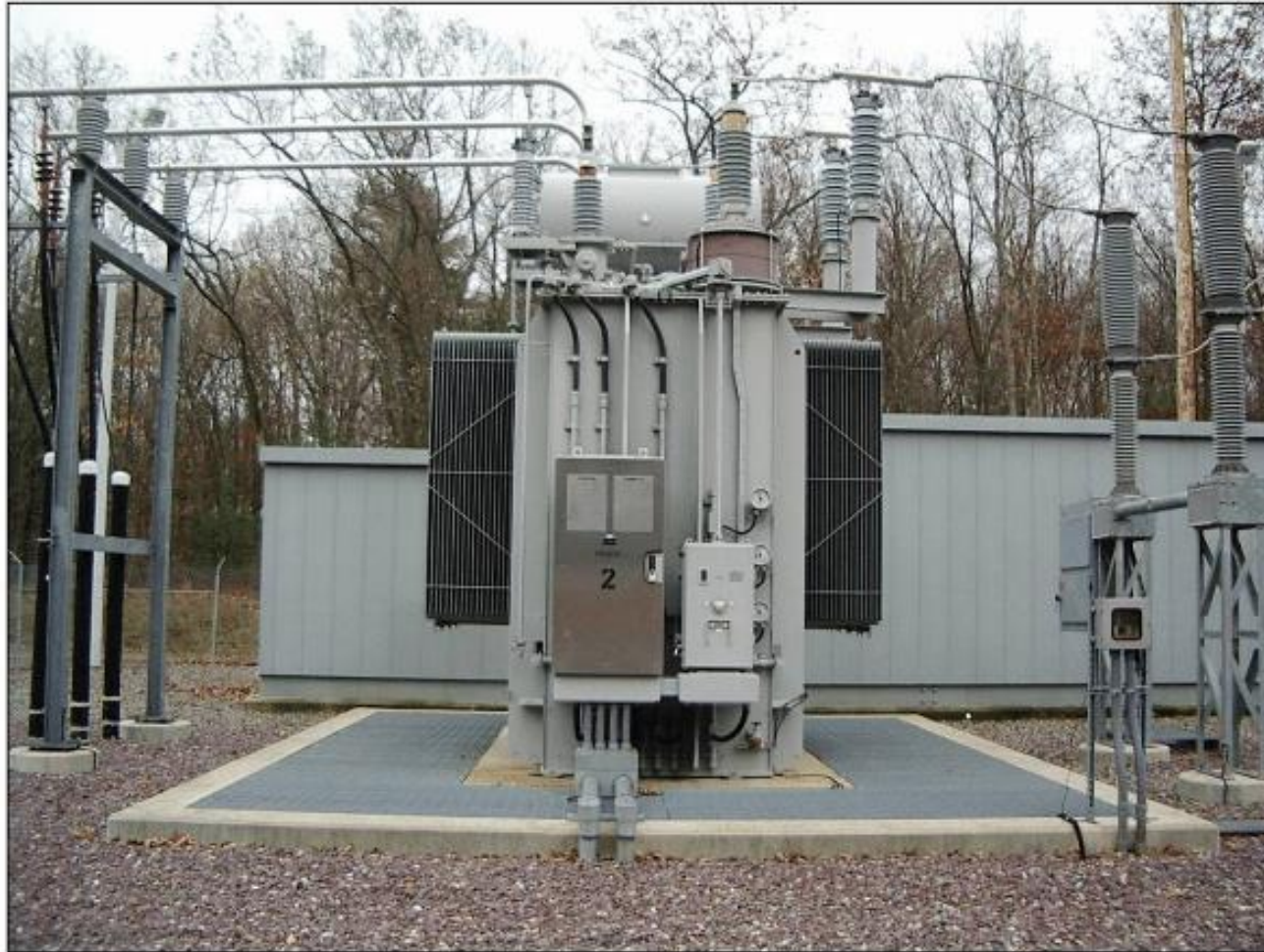
Amtrak's North End Electrification
