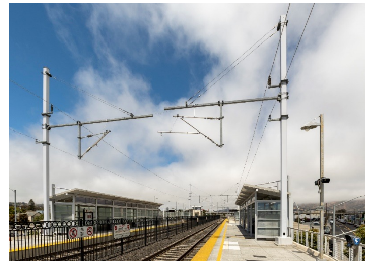
Overhead Catenary System
