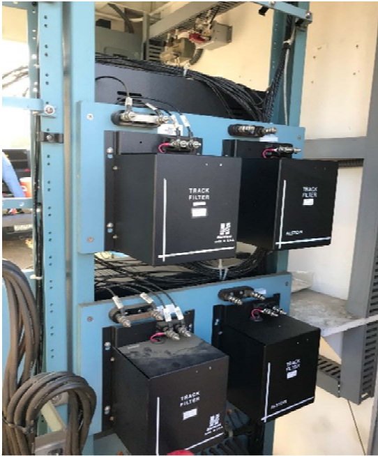
Photo 1 - New advance signal preemption equipment
