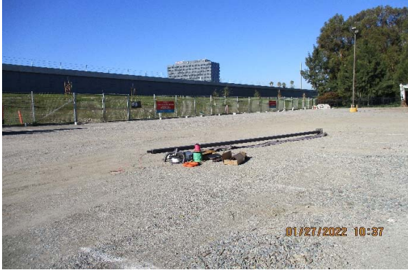
Photo 1 - 25th N Yard Lighting Pole
