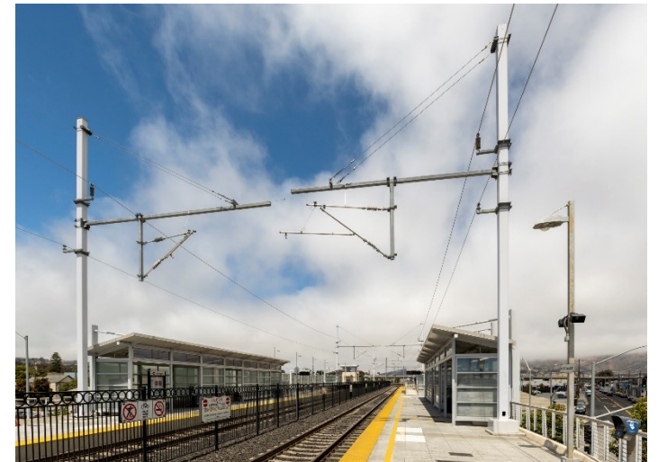
Overhead Catenary System
