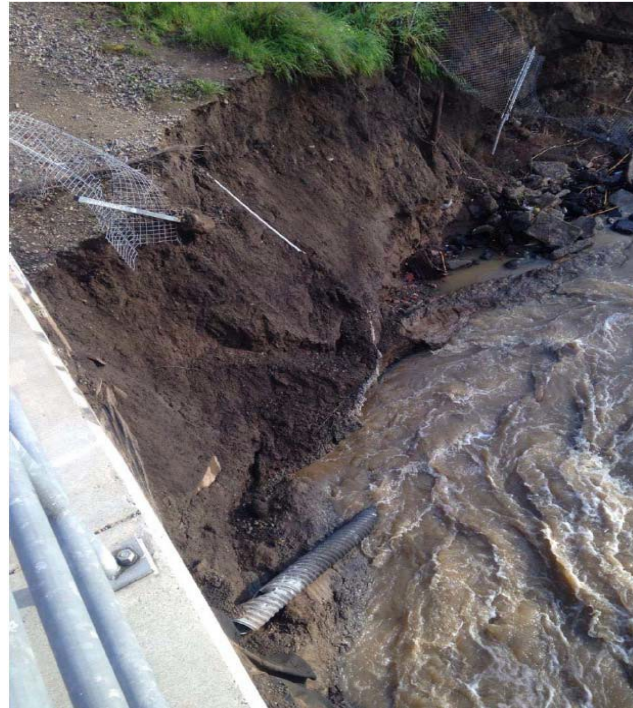
MT-2 Bank Failure
