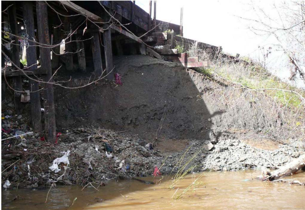
MT-1 Bank Failure
