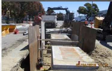
Splice boxes on Grand Avenue
