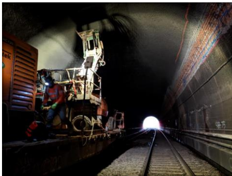
Tunnel 4: OCS Anchor Bolt Installation using Template (left) and Exposed Brick from Notching (right top)
