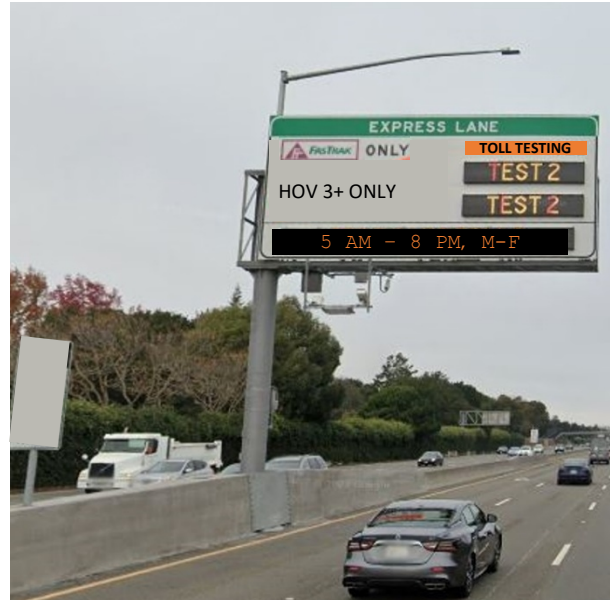
Toll Equipment Testing
