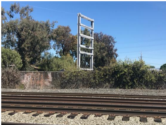
TPS2 Isolation Gantry
