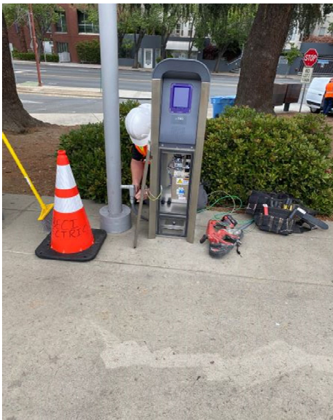
Photo 3 - Palo Alto Prototype Inside
