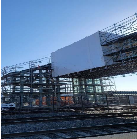
Photo 1 - Platform view of scaffolding containment system
