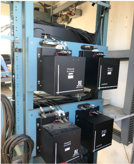
Photo 1 - New advance signal preemption equipment
