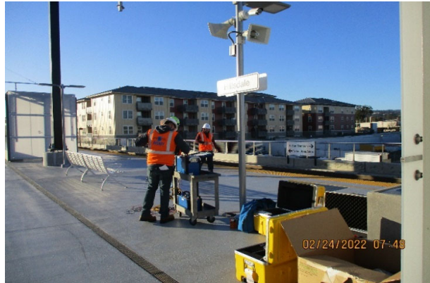
Photo 2 - OCS Grounding Testing.
