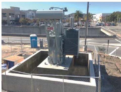
Paralleling Station 4 Hillsdale Station
