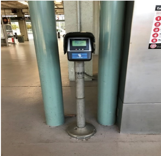
Photo 1 - Old Clipper CID removed via Change Order
