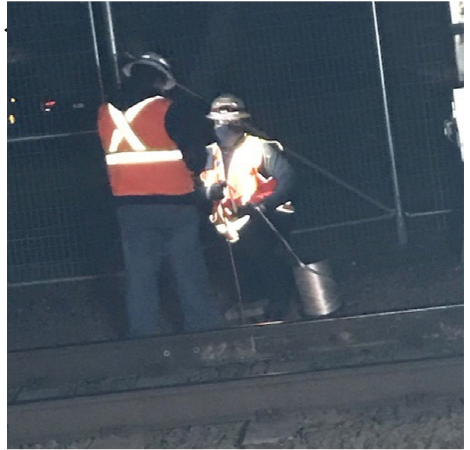
Photo 2 - Workers putting in new signal wires for the train detection in the rail
