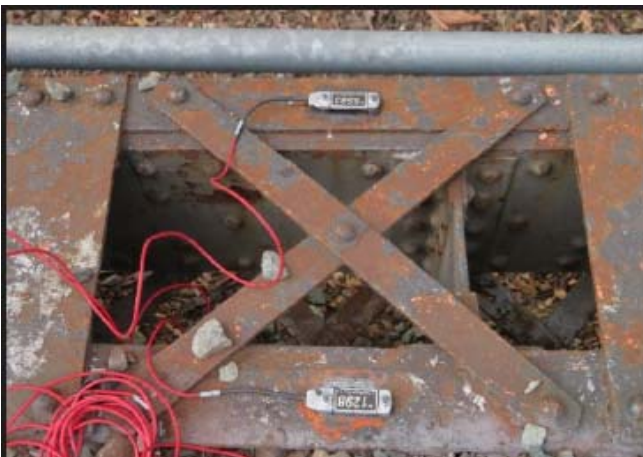
Photo 3 - Strain Gauge on Horizontal Chord
