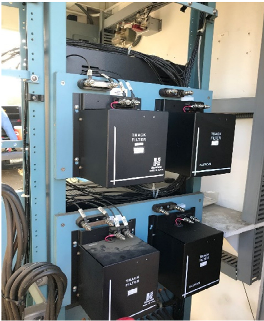
Photo 1 - New advance signal preemption equipment
