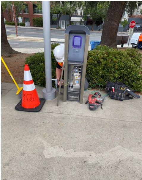
Photo 3 - Palo Alto Prototype Inside
