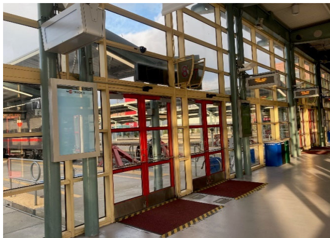
Photo 4 - Doors 5, 6, 7 and 8 APC
