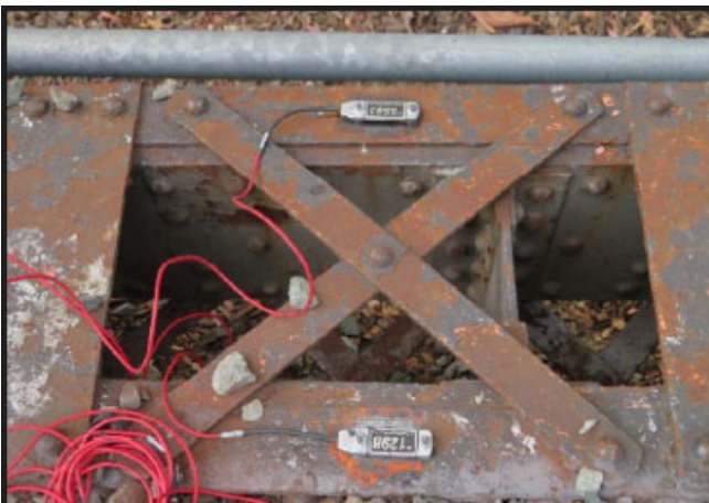
Photo 3 - Strain Gauge on Horizontal Chord
