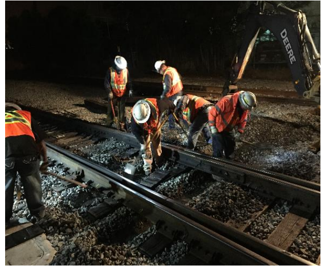
Crews replacing worn switch ties near Control Point (CP) Bird at San Jose Diridon Station
