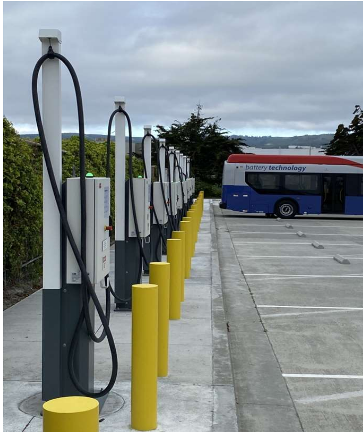
North Base BEB Interim Chargers
