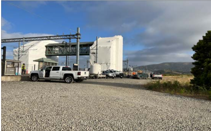
Photo 1 - West Side Containment System
