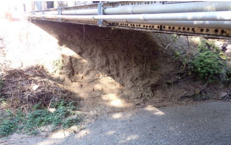
Photo 3 - North bank Erosion
