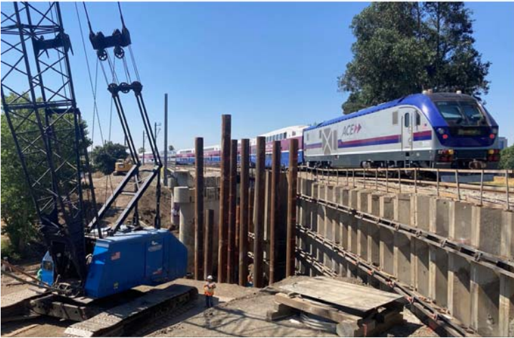
Photo 1 - Cast-in-Concrete-Shell (CISS) piles being installed for MT2 pier 5 while MT1 remains in service
