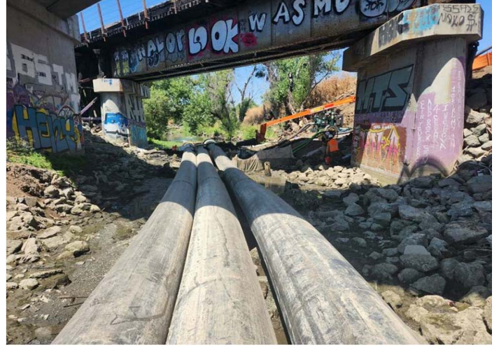
Photo 2 - Implementation of a temporary river diversion system to allow dewatering of the site
