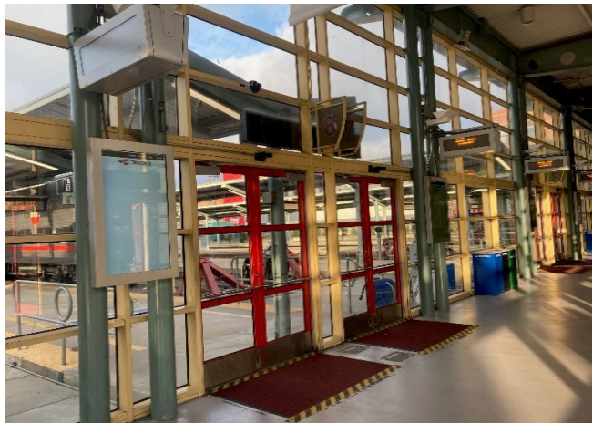
Photo 4 - Doors 5, 6, 7 and 8 APC
