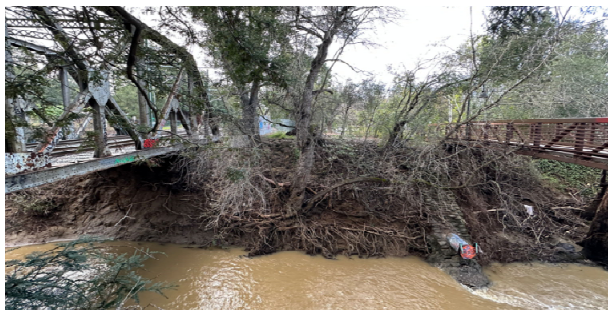
Photo 1 - Eroding north bank of the San Francisquito Creek under Caltrain's bridge (left) and the Alma Street Bicycle Bridge (right)
