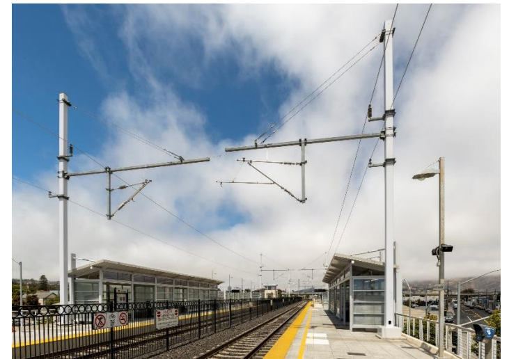
Overhead Catenary System
