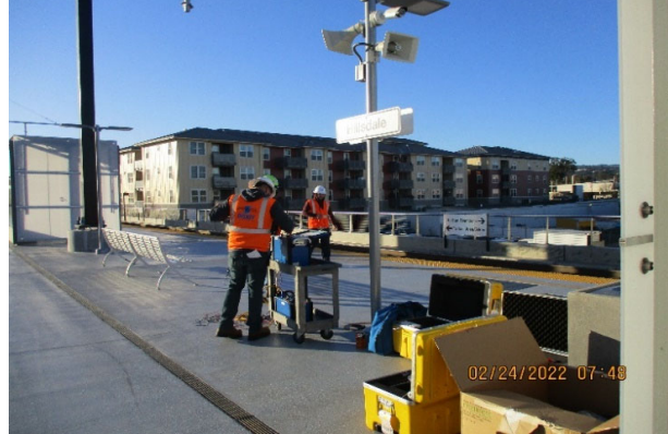
Photo 2 - OCS Grounding Testing.
