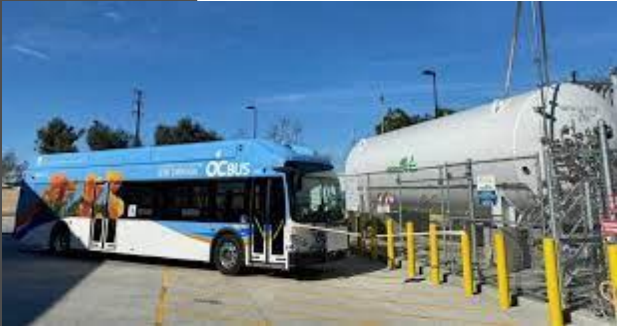
Hydrogen Storage & Fueling Station
