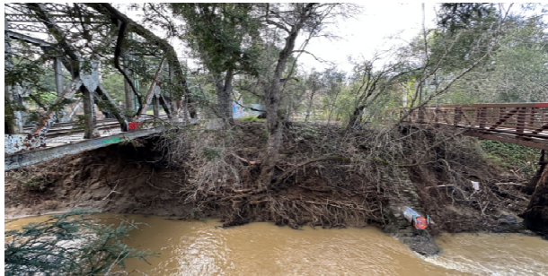
Photo 1 - Eroding north bank of the San Francisquito Creek under Caltrain's bridge (left) and the Alma Street Bicycle Bridge (right)
