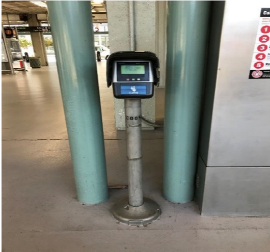
Photo 1 - Old Clipper CID removed via Change Order
