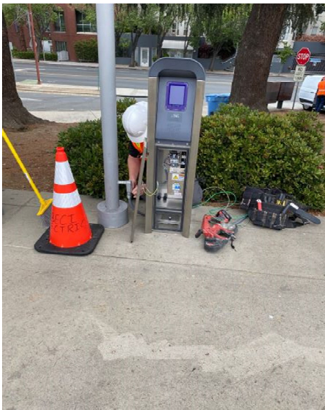
Photo 3 - Palo Alto Prototype Inside
