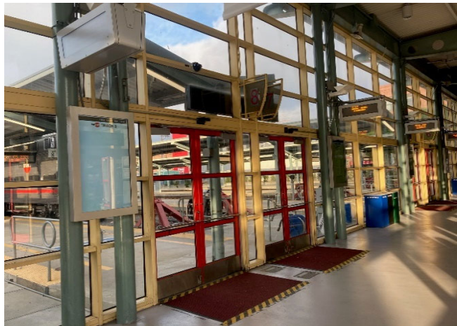
Photo 4 - Doors 5, 6, 7 and 8 APC
