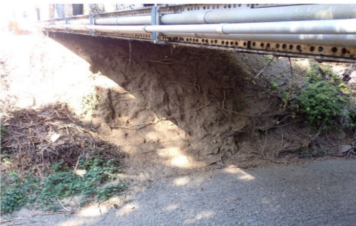
Photo 3 - North bank Erosion
