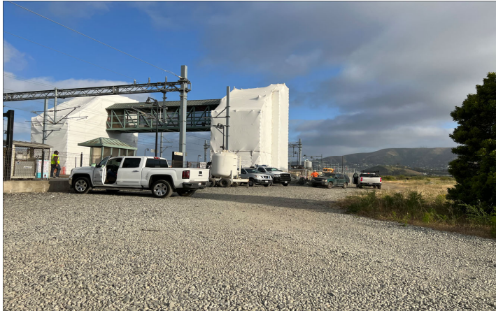
Photo 1 - West Side Containment System
