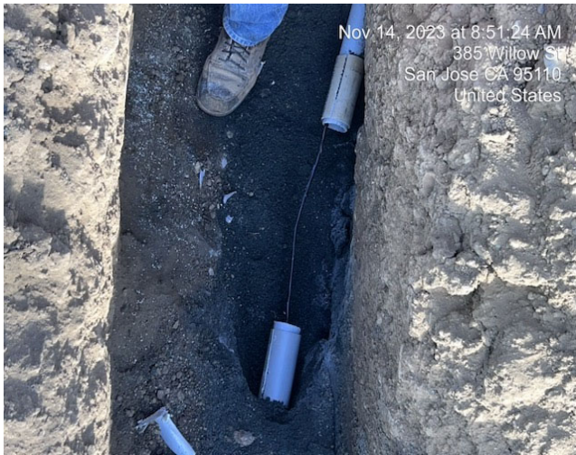
Photo 1 - Trenching and Conduit for the electrical power cable to the Broadband Radio.
