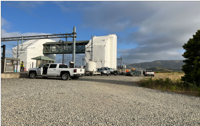
Photo 1 - West Side Containment System
