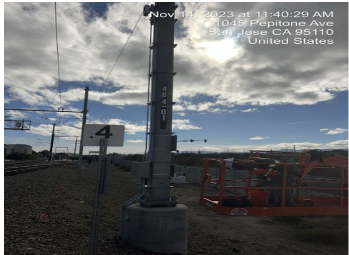
Photo 2 - Broadband Radio mounted on the OCS pole.
