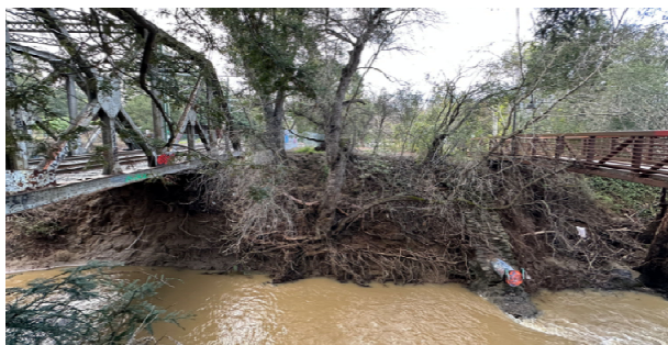
Photo 1 - Eroding north bank of the San Francisquito Creek under Caltrain's bridge (left) and the Alma Street Bicycle Bridge (right)
