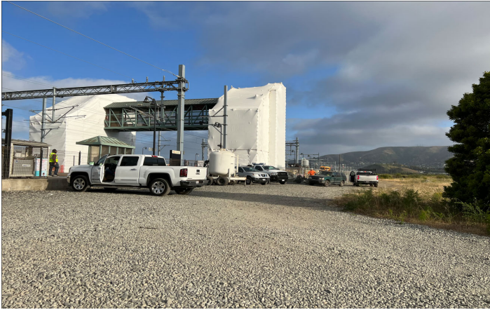
Photo 1 - West Side Containment System
