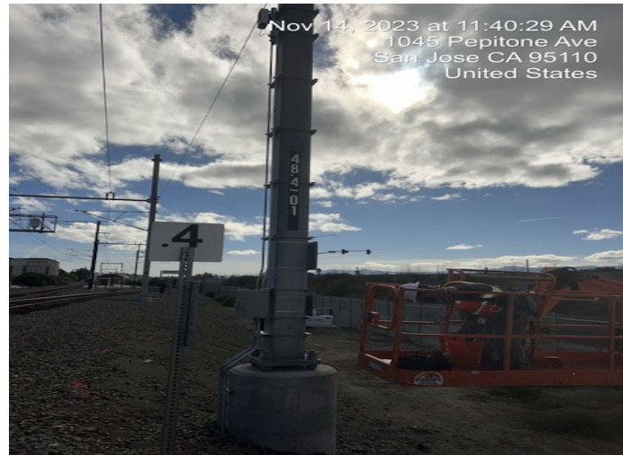
Photo 2 - Broadband Radio mounted on the OCS pole.
