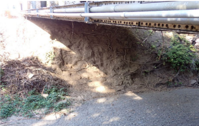
Photo 3 - North bank Erosion
