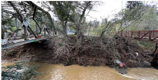
Photo 1 - Eroding north bank of the San Francisquito Creek under Caltrain's bridge (left) and the Alma Street Bicycle Bridge (right)
