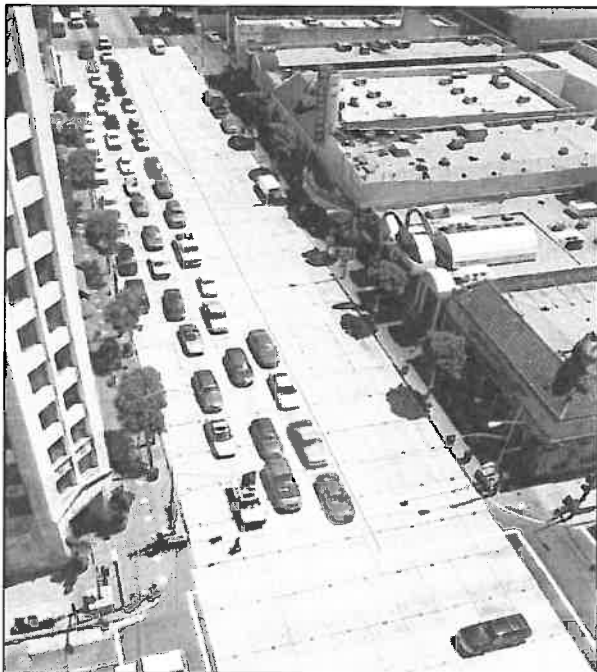
Figure 2: Traffic Decking for the Red Line at Hollywood Blvd./Highland Ave. in Los Angeles
