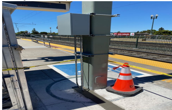
Photo 4 - Radio box installed on OCS pole at San Carlos station
