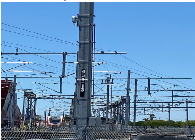
Photo 3 - Radio on OCS pole at the train maintenance facility
