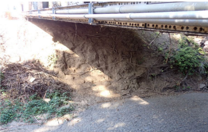
Photo 3 - North bank Erosion
