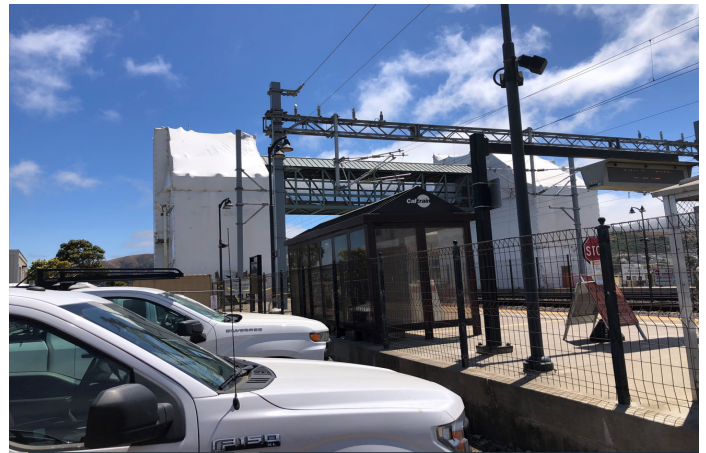
Photo 2 - East Side Containment System
