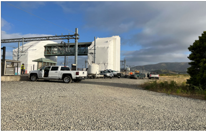
Photo 1 - West Side Containment System
