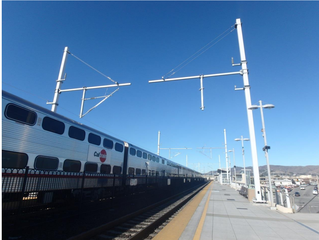
Overhead Contact System
