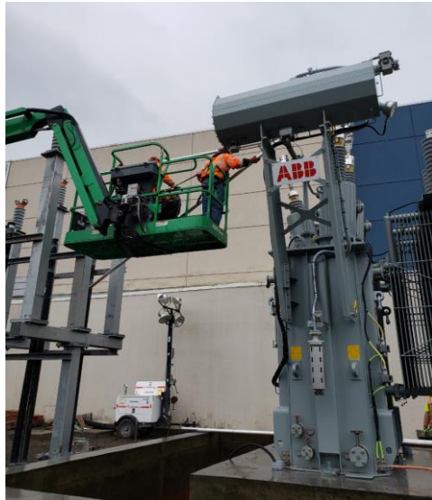
BBII electricians running bus conduits at the transformer and bending the conduits to size for installation at PS-5.
