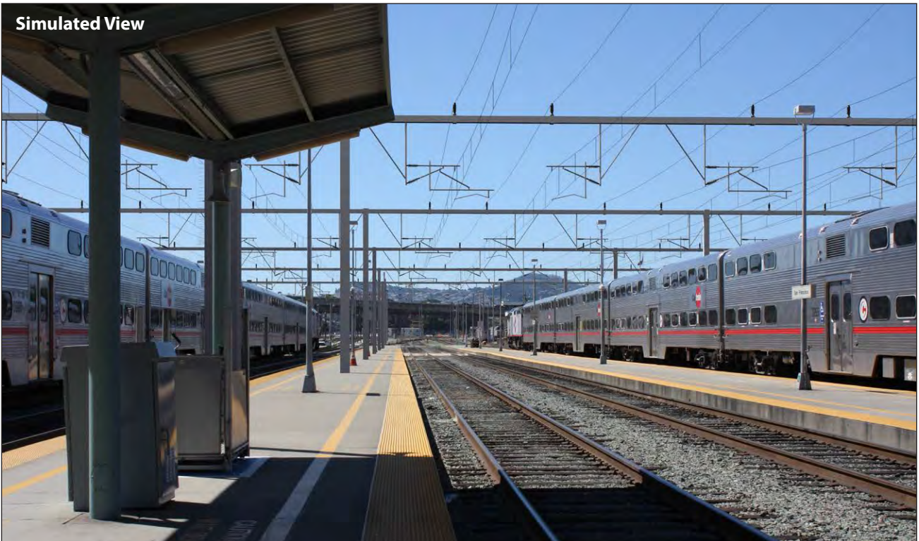
Looking southwest down the rail corridor with the OCS system, as seen from the San Francisco Caltrain Station at 4th Street
