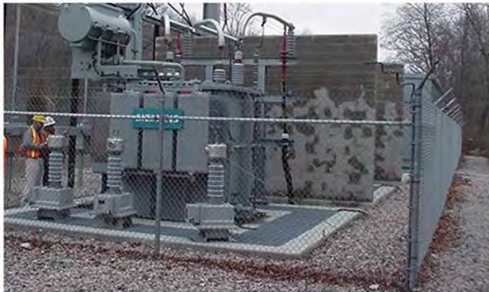
Auto-Transformers with Fire Walls
