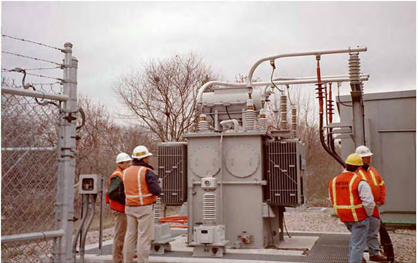
Amtrak's North End Electrification
