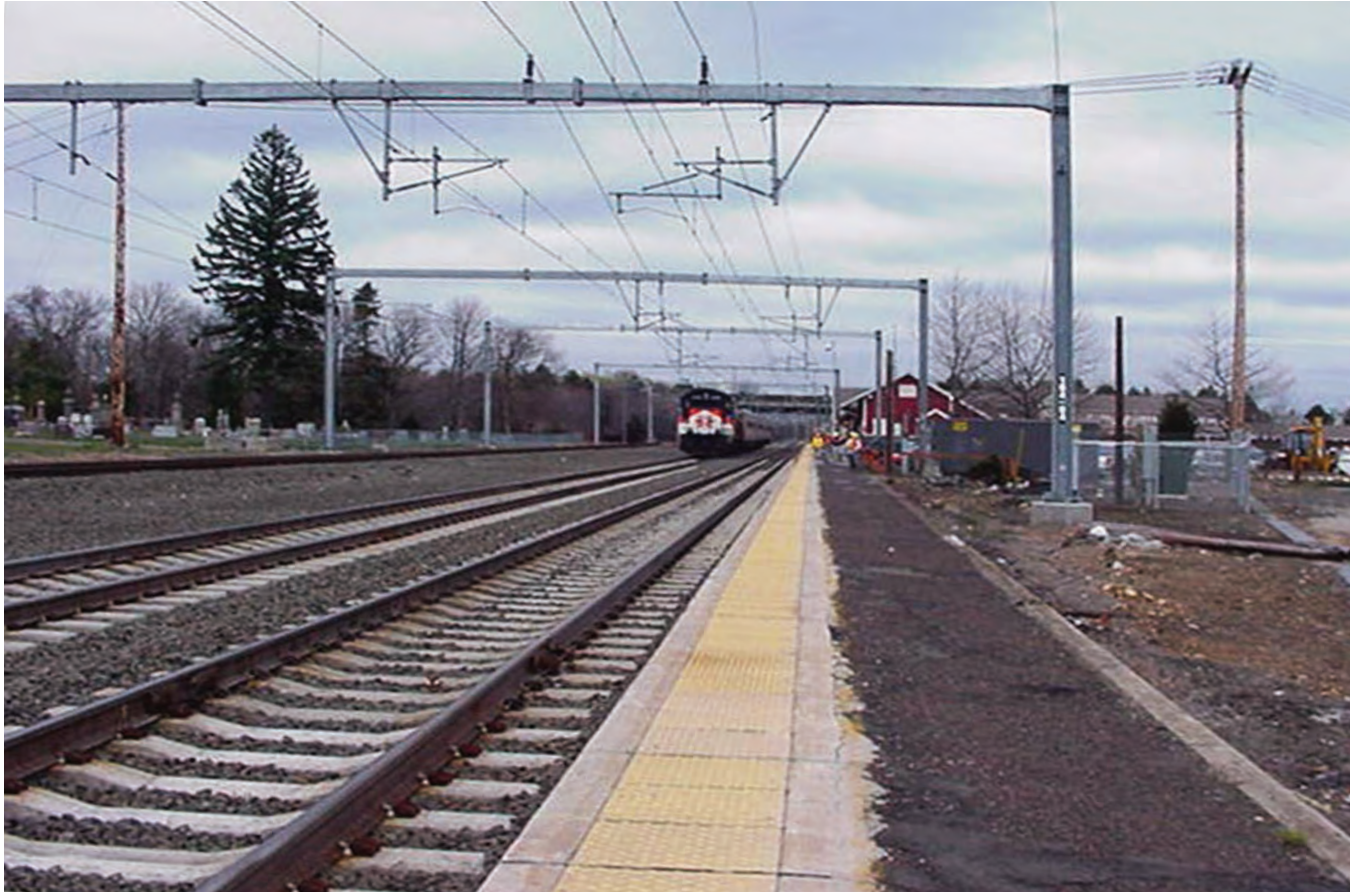
Amtrak's North End Electrification
