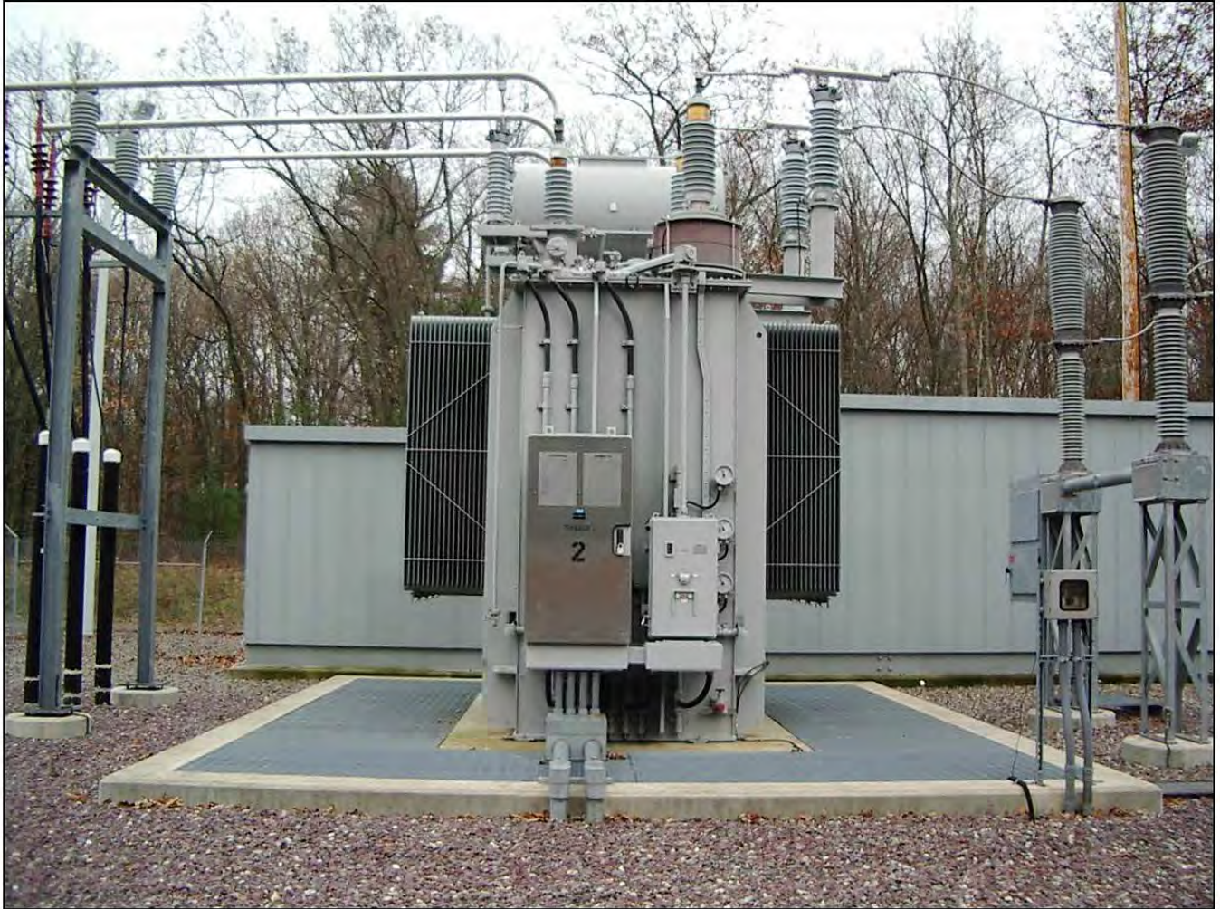
Amtrak's North End Electrification
