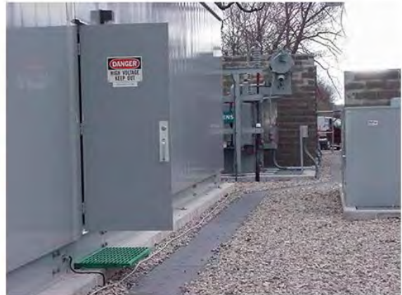
Control Building and Auto-Transformer
