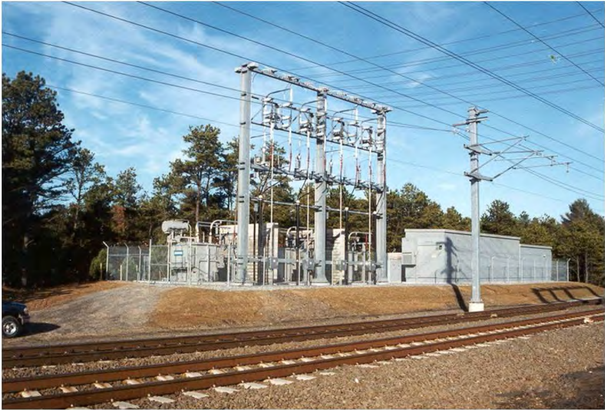
Amtrak's North End Electrification
