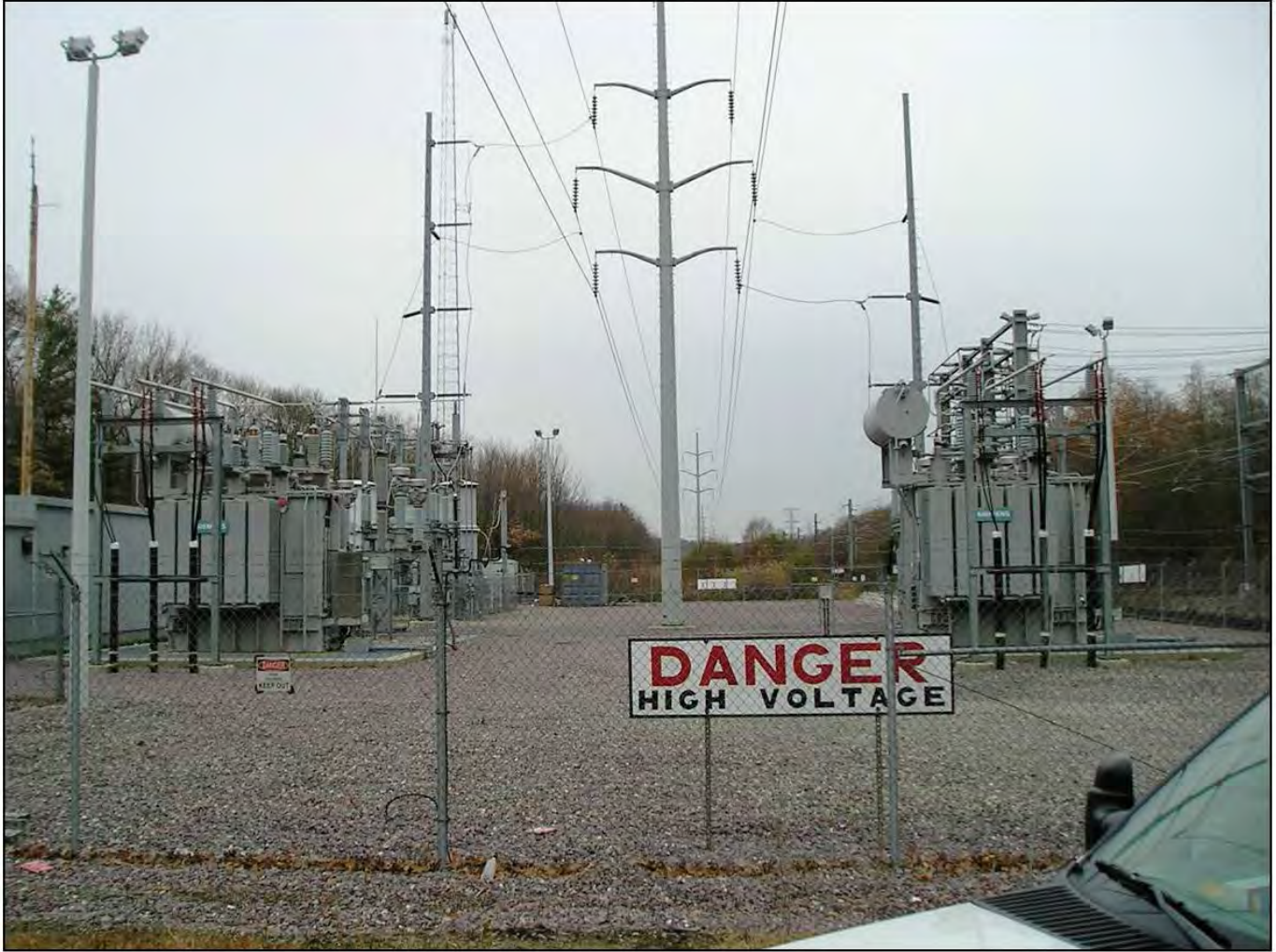
Amtrak's North End Electrification
