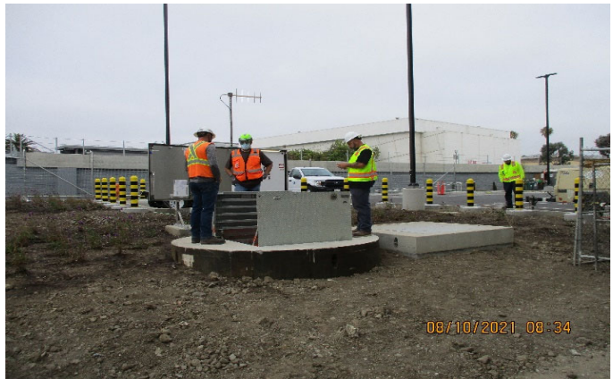
Photo 2 - Pump Station Testing
