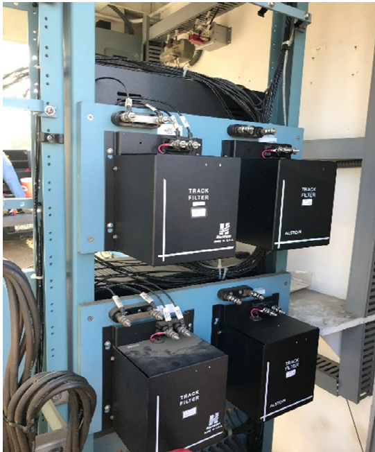
Photo 1 - New advance signal preemption equipment
