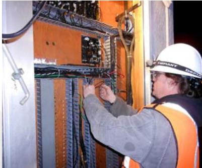
Installing new wires at the rear of the entry rack
