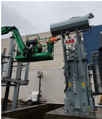
BBI electricians running bus conduits at the transformer and bending the conduits to size for installation at PS-5.
